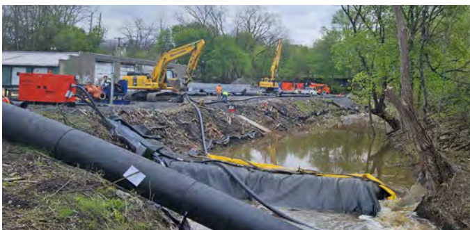
Left- A temporary dam allowing water to drain as Severson stages equipment in the floodplain.
