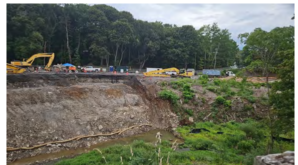
Right- Excavators staged at Upson Park as creek and floodplain remediation continues.
